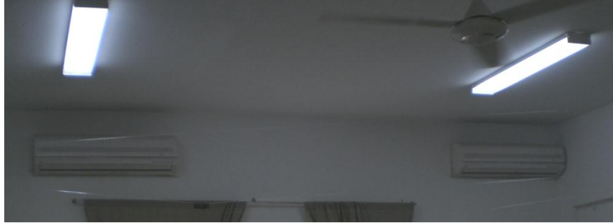
Figure 4-8: AC Units in School-A (Taken by the author).
