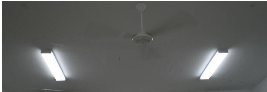
Figure 4-25: School-A Covered Luminaries (Taken by the author).
