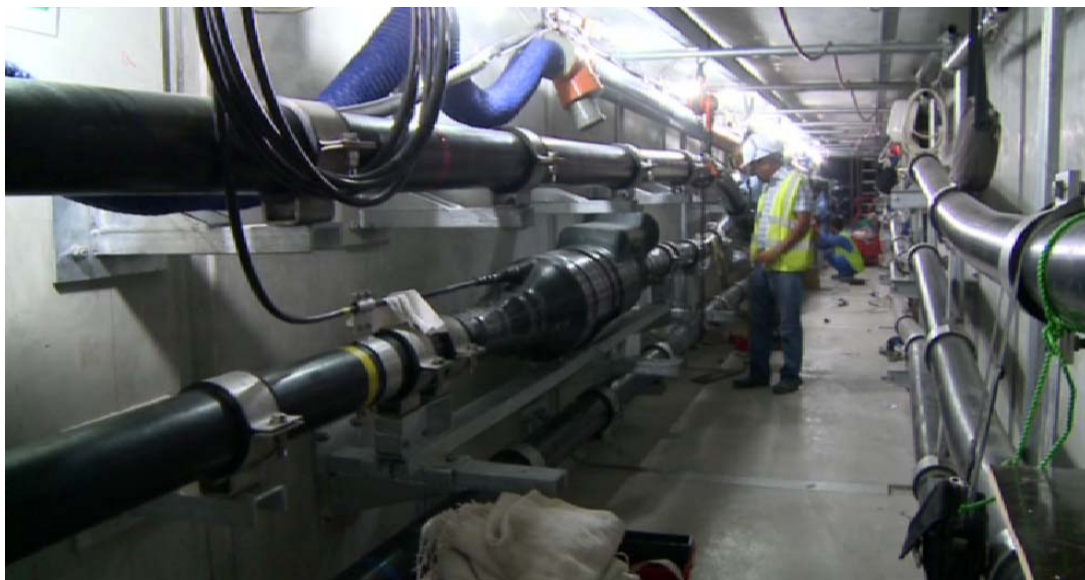
Picture -1: 400kV Cables – Transmission Lines (DEWA/Nexan, 2011)
